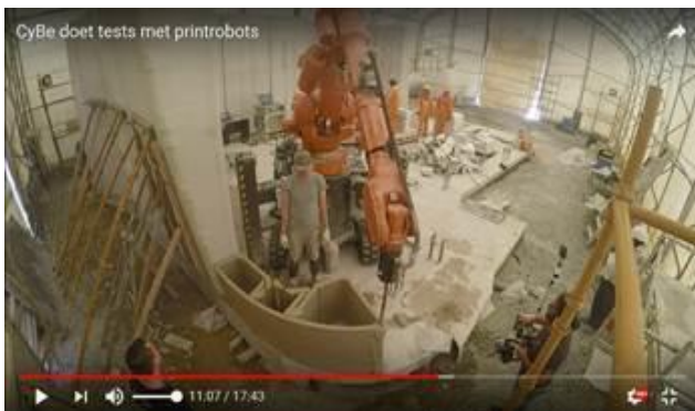
Excess materials being placed around corners due to slowing down of the print speed at the corners
